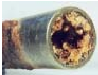
Corroded Galvanized pipe prior to ACE DuraFlo restoration.
